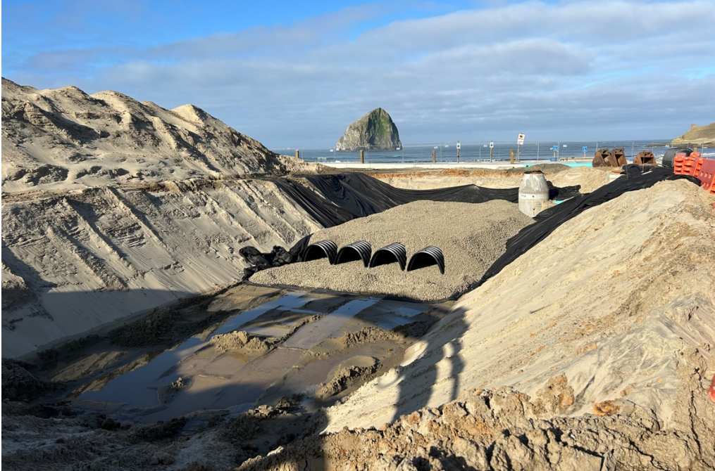
New Stormwater Management System
